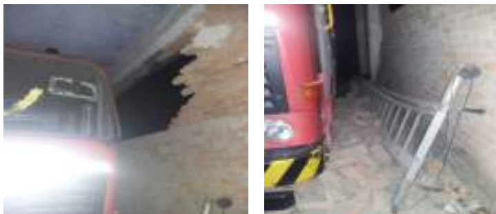
Fire & Emergency Services, Tarapur, Silchar side wall damage during Earthquake.
